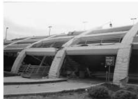
Fig. 1: Parking structures that collapsed during the 1994 Northridge earthquake, California State University,
