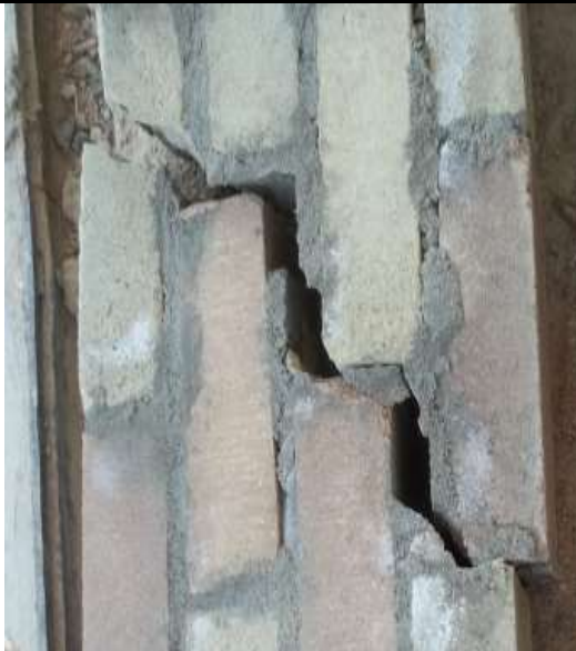
Fig.17: Crack Pattern (Normal to Bed Joint)
