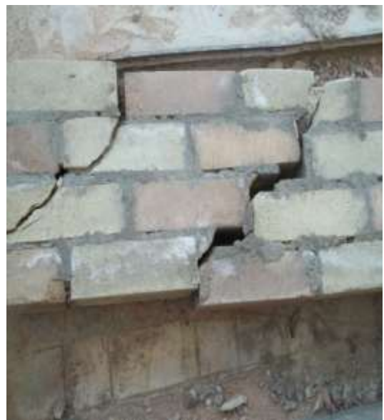
Fig.16: Crack Pattern (Parallel to Bed Joint)
