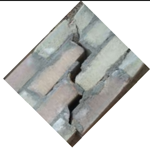
Fig.14: Combined Cracks through head and bed joints
