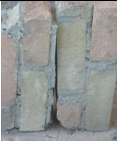
Fig.13: Crack Pattern (Normal to Bed Joint)
